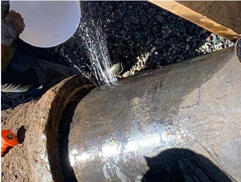
Water main leak
