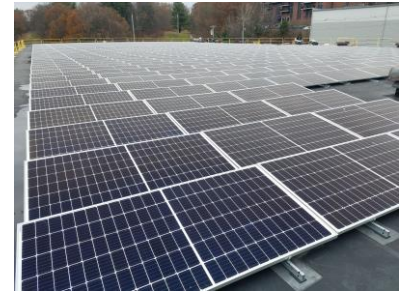
Solar Panels installed at Stoneham Ice Arena
